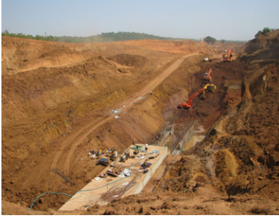
Fig. 11. 2: An Inter-basin irrigation canal being dug at Kankumbi village, headwater region of Mhadei in Karnataka state
