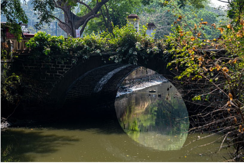
Fig. E.10: Sewage emptying out into the river. Source: Shrinivas Ananthanarayanan/Gasper D'Souza Collection.
